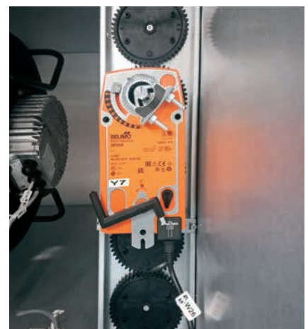
Figure 54: Actuator for the fresh air and exhaust dampers.
