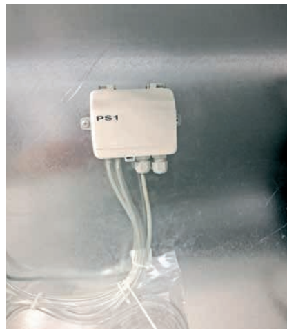
Figure 50: Pressure sensors unit with two differential pressure sensors. In CompAir it is used for measuring pressure in duct and also for measuring air flow of inlet and outlet fans. Communication with controller is via EXOline communication.
