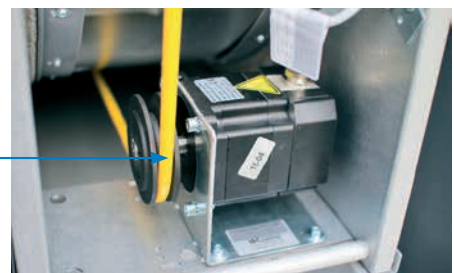
Motor with belt drive
