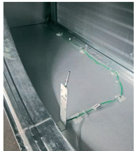
Figure 53: Temperature sensor for inlet air temperature. It has to be connected in the connection box located behind supply fan (green connector – see Figure 54
