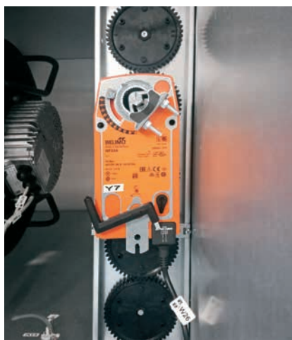
Figure 55: Actuator for the fresh air and exhaust dampers,
